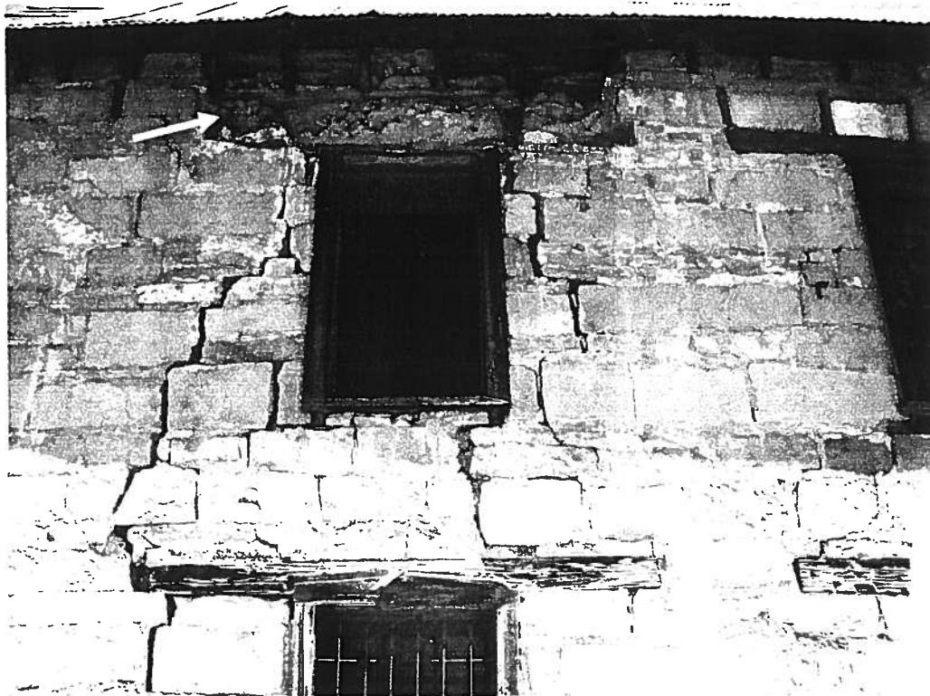
Photo 6. Lintel beams are rotted and missing on the north wall [5/22/03].
