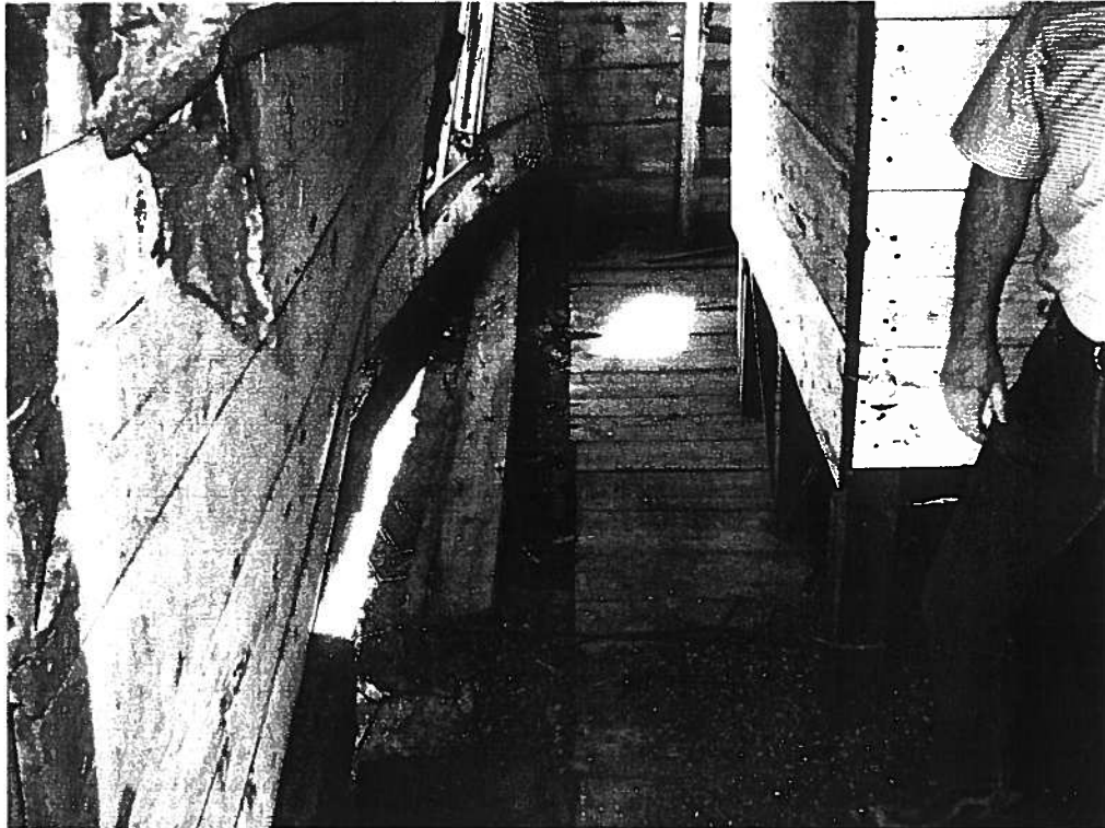
Photo 9. Third floor end all bowed out due to wall settlement and rotation [5/22/03].
