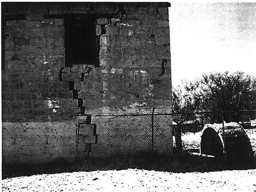
Photo 12. Stone cracking on the East end of the south wall [5/22/03]
